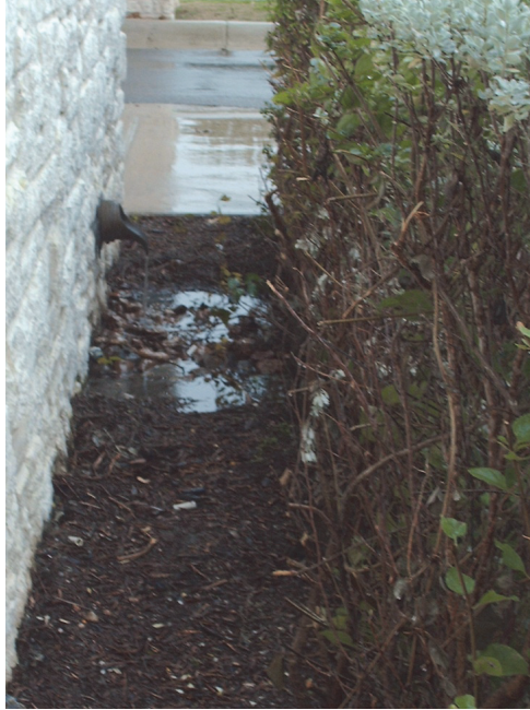
Fig. 1. Site drainage violated code and, held water against the building.
