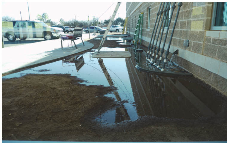
Fig. 11. Improper site grading.
