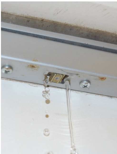
Fig. 4. Water entering the building because of inadequate flashing.
