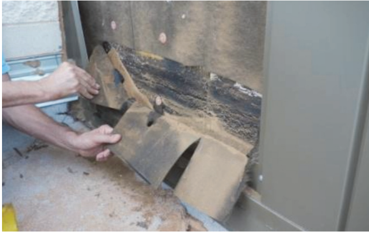
Fig. 14. Infiltration of dirt and moisture under parapet wall.
