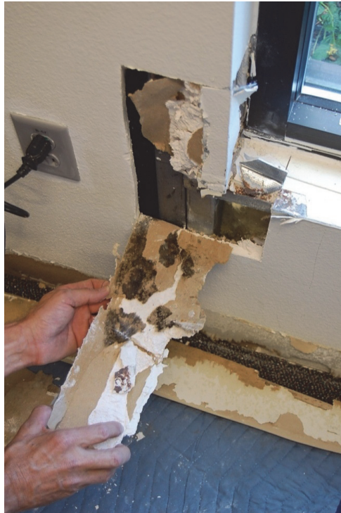
Fig. 3. Mold caused by moisture in the wall cavity.
