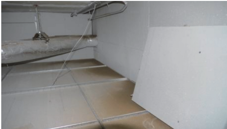
Fig. 15. Infiltration of dirt into the attic space above lay in ceiling.
