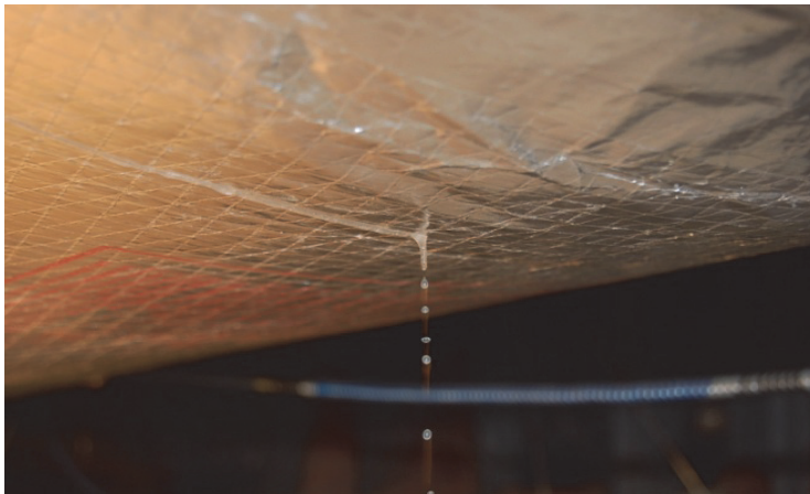
Fig. 10. Water running out of insulation.
