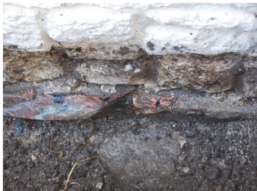
Fig. 2. The copper-coated base flashing at the applied masonry veneer wall terminated below grade and therefore did not allow for the water to drain.
