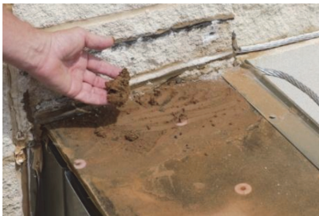
Fig. 13. Infiltration of dirt and moisture under parapet cap.
