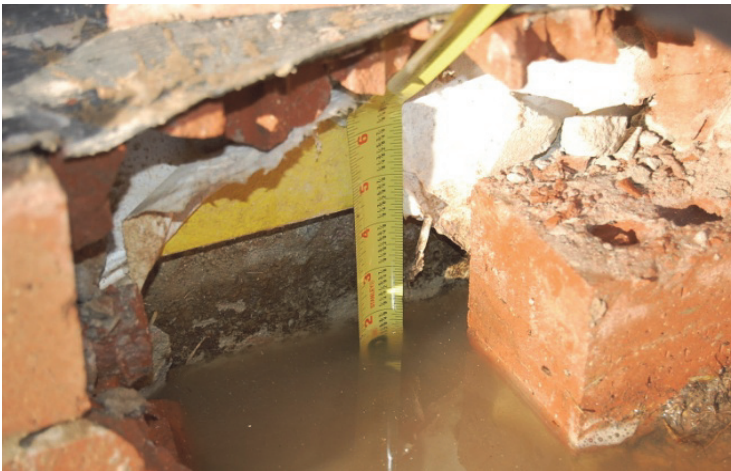
Fig. 9. Water standing inside the wall cavity.
