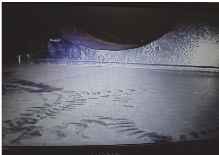
Fig. 16. Tracks of robotic camera in the dust of the HVAC ductwork.
