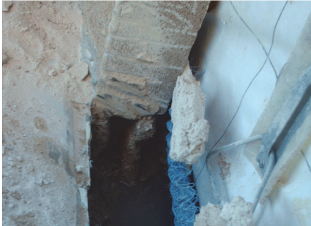
Fig. 12. Water standing inside wall cavity.
