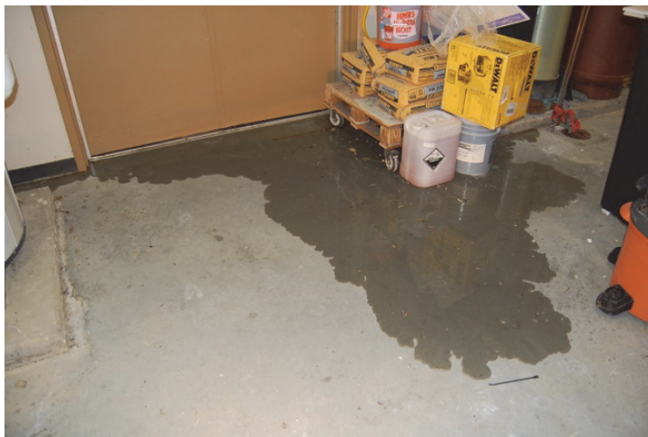
Fig. 7. A flawed detail at the base of the building compounded the threat to the building posed by standing water.
